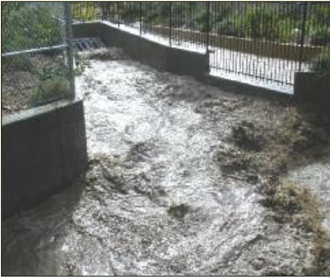
Constructed upstream inlet being tested during a January 2010 storm
