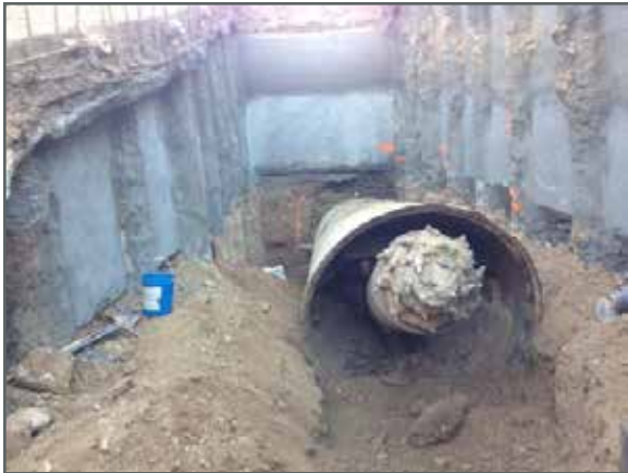
Figure 11. Upper tunnel Rotohead excavator as it emerges into the upstream inlet structure.
