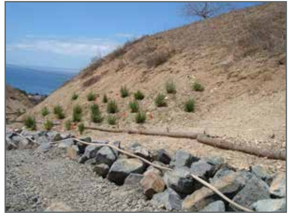
Figure 15. San Ramon Canyon adjacent to Tarapaca Landslide with rip rap rock bottom and landscaping in progress.
