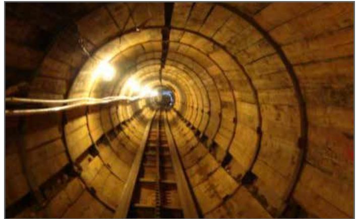
Figure 12. Completed upper rib and lagging tunnel prior to installation of the 54-inch storm drain pipe.
