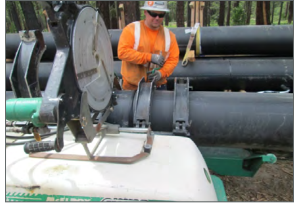
Figure 7: Fusion welding for the NTPUD Dollar Hill Force Main project. This joint is currently in the cooling phase.
