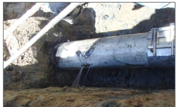
Figure 5: Existing leak in PVC force main
